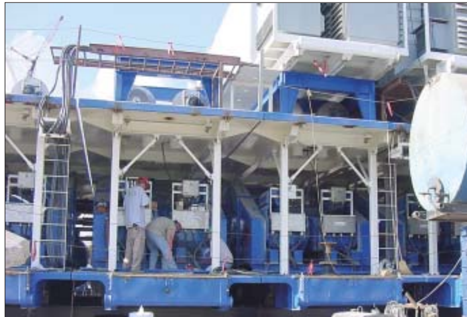
Power distribution equipment sits above the power generation sets, during construction in New Iberia, La. The drilling services module or utility train contains 50 skid equipment packages that must stack together for the module to fit within a reasonable space at the drilling location (Fig 10). Photo courtesy of ExxonMobil Corp.
