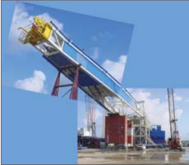
Parker Rig No. 262 mast rests on scaffolding in the construction yard at New Iberia, La. The rig's drawworks will upright the mast from the scaffolding, which will be the rig-up method at the Sakhalin drilling location (Fig. 11). Photo courtesy of ExxonMobil Corp.
